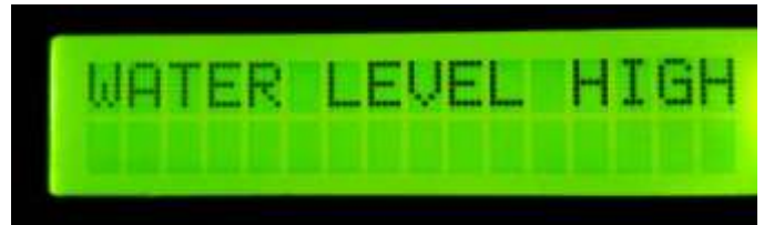
Figure 9.Displays status of water level in tank
